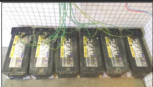
Fig. 2: Stationary battery bank used
